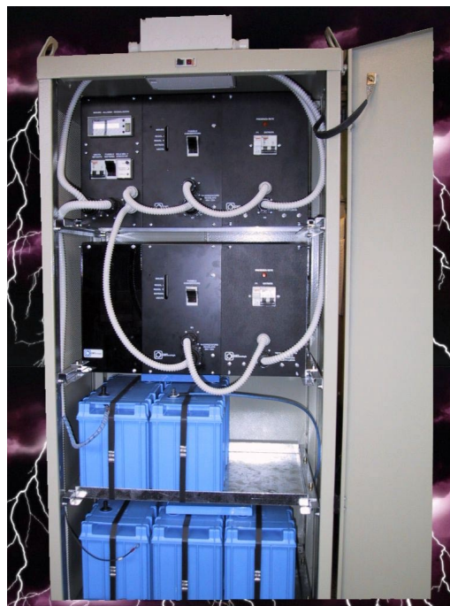
Power energy station SETB 2000-6-R
